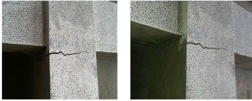
Figure 11. Cracking under concrete beams. Source: [1]
