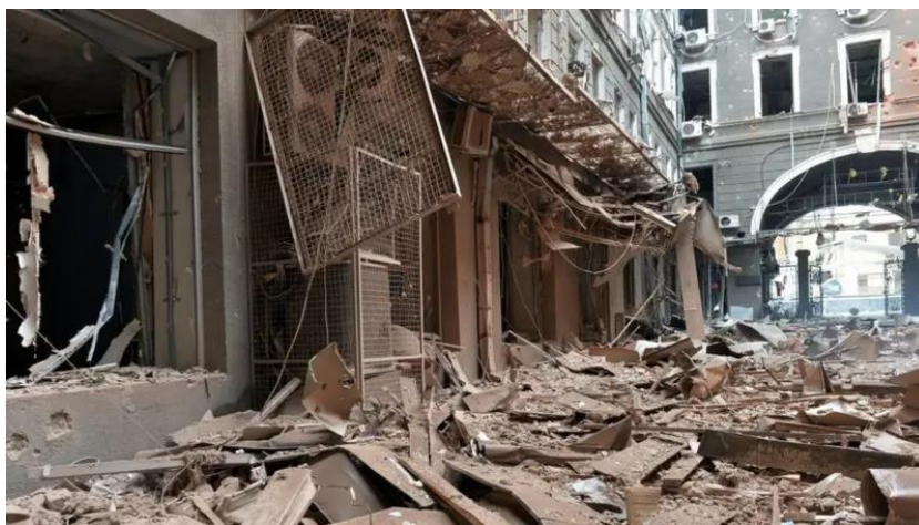
Image 2. "Damage to the entrance of a building in Kharkiv, caused by the Russian attack"
