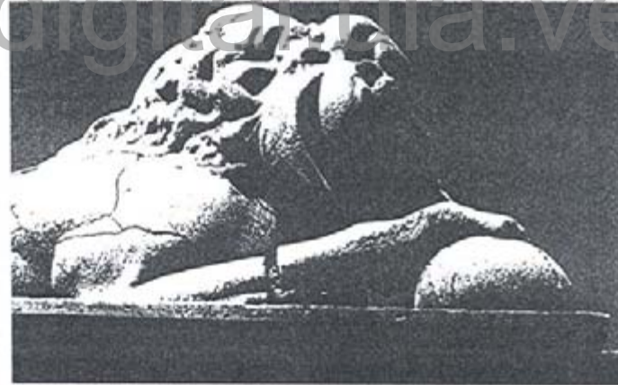
Mortar lion figure, showing carbonation problem, located at one of the bridge ends.
