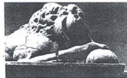
A mortar lion located at the end of a concrete bridge suffered severe damage from carbonation. See p. 56 for an article that discusses corrosion and carbonation effects on historic structures and suggests guidelines for structural refurbishment.
