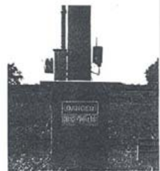
A wireless remote monitoring device was installed at a refinery site for field equipment monitoring and data transmission. An article beginning on p. 26 describes the technology.
